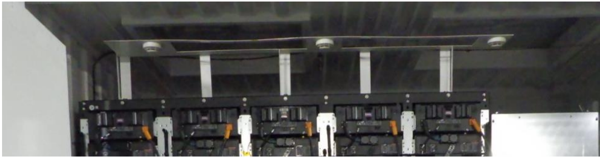
Figure F5 – Photo of the smoke detector installed above the rack
