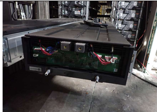
Post Test – Front View of Module 9
