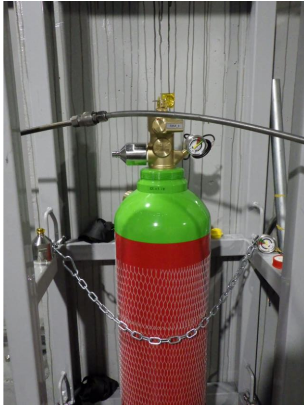
Figure F2 – Photo of Novec 1230 Cylinder
