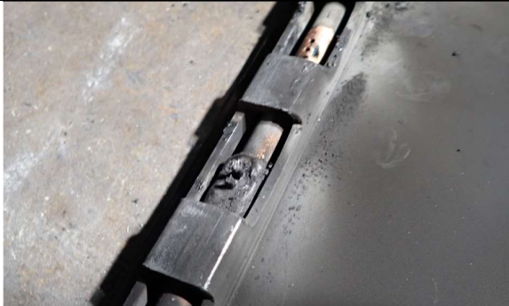
Post Test – View of the NOVEC Piping
