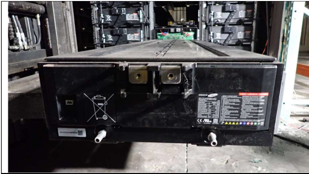
Post Test – Front View of Module 11
