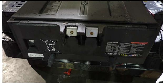
Post Test – Rear View of the Initiating Module
