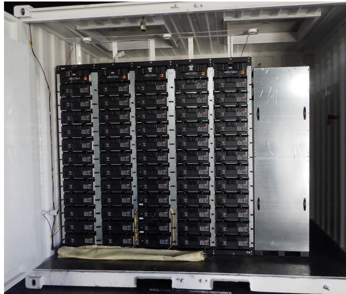
Figure 1 – Picture of the units in the container
