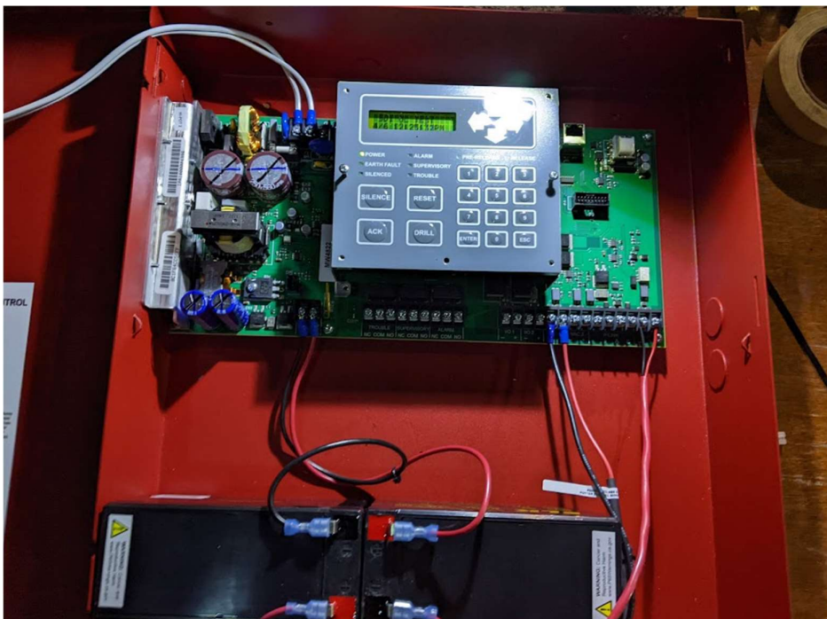
Figure B5 – Fire Panel System – Connected to the NOVEC Release System
