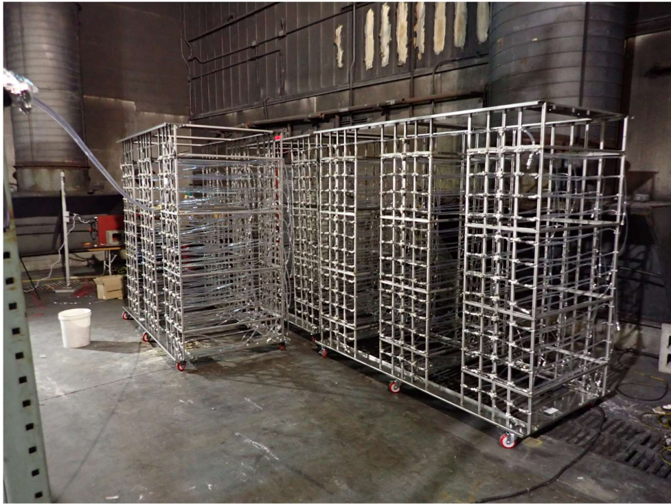
Figure B7 – Dummy Racks with NOVEC Piping 6
